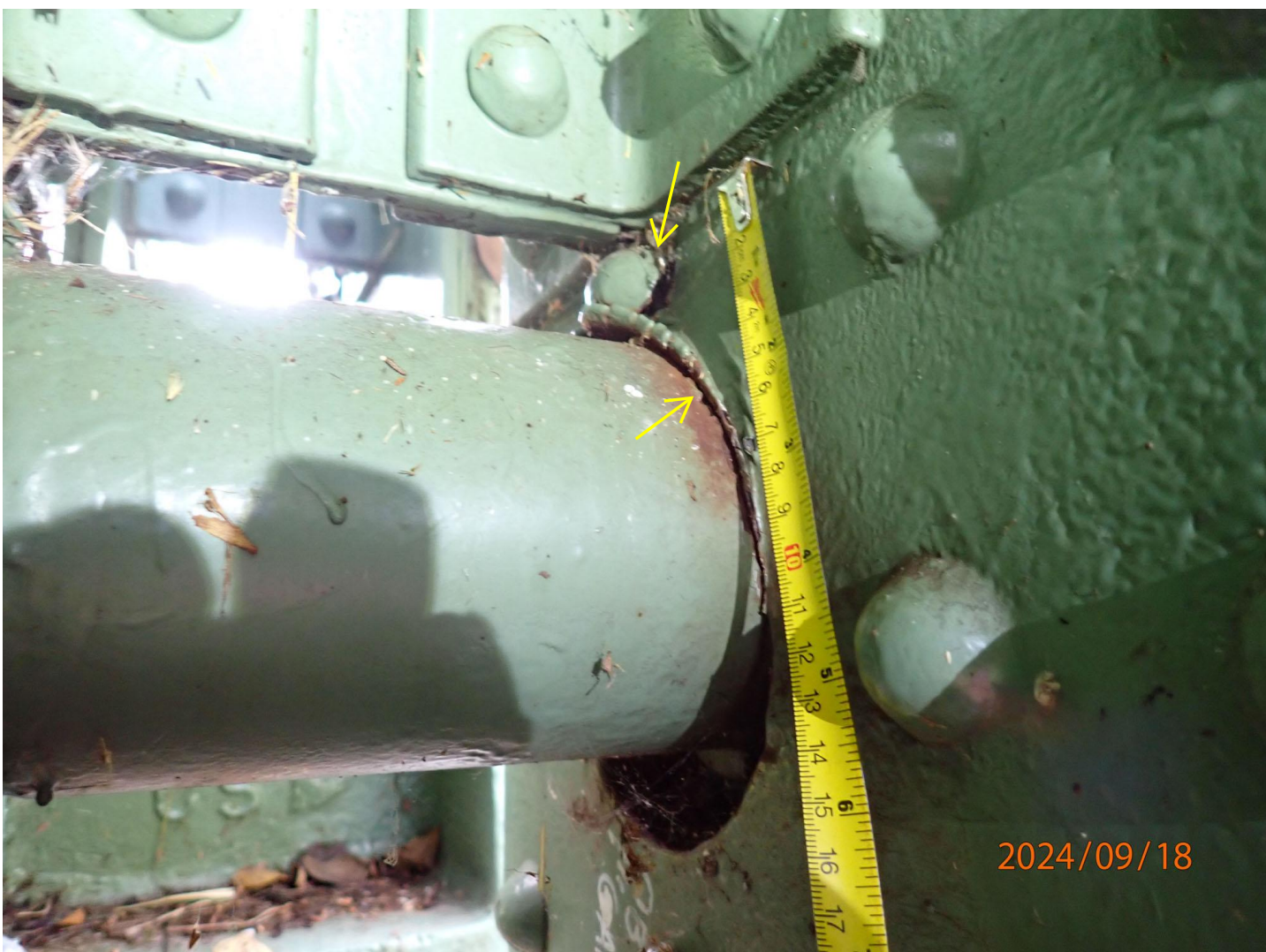
Pratt Truss 1, L0 bearing Close-up north side with deformation of plate, plus rivet head failing.
